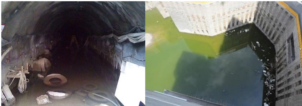
Fig. 1. An example of rising water level (wastewater) in the projects of the city center of Mashhad (Ghahremani et al., 2017)
